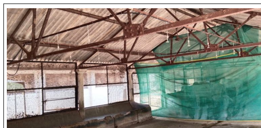
Plate 2: Installation of fogger assembly for creation of cooling effect inside the dairy shed.
