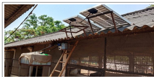
Plate 1: Solar power assisted cooling system.
